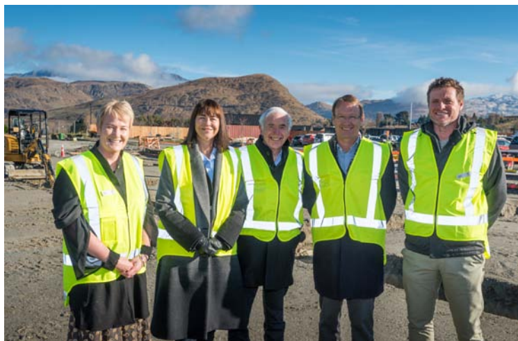
Investment Committee (June 2020): (L to R) Susan Finlay, Linda Robertson, Sir Eion Edgar (chair), Mark Taylor and Lindsay Breen viewing the construction of the Southern Cross Central Lakes Hospital, due for completion in late 2021
